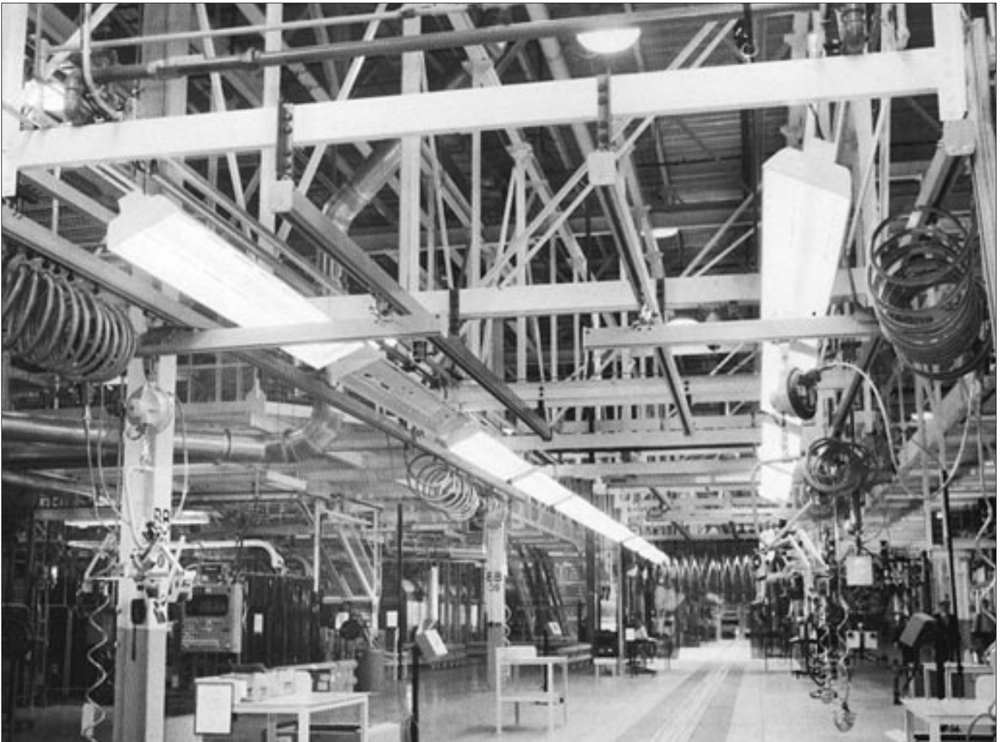
BODY SHOP TOOLING AREA ETA-4 BRIDGE CRANE SYSTEM
